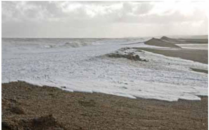
The sea overspilling the seawall at Cley in March 2007.
