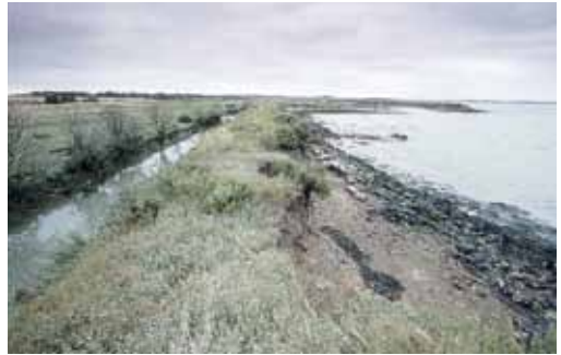
An eroding seawall at Orlands, Essex.
